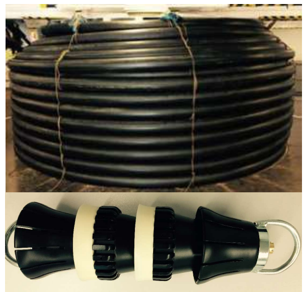
Figure 8. “Sonic head” used to install 646 m of 82 mm power cable into 125/102 mm duct coiled with 2 m radius
